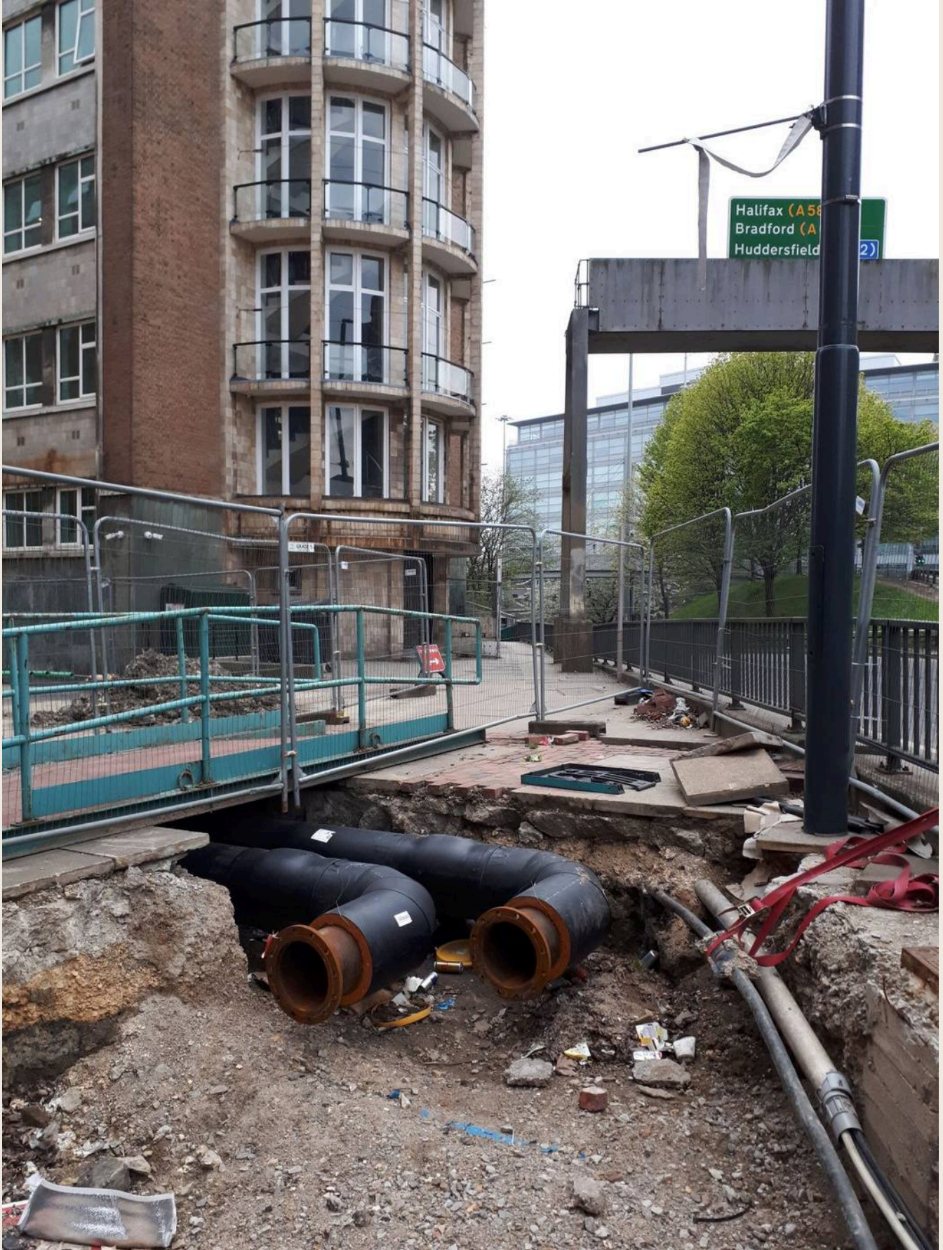
FIG. 10 · DISTRICT-HEATING PIPEWORK, LEEDS · PHOTO: STEPHEN CRAVEN / WIKIMEDIA COMMONS · CC BY-SA 2.0. Source and licence
