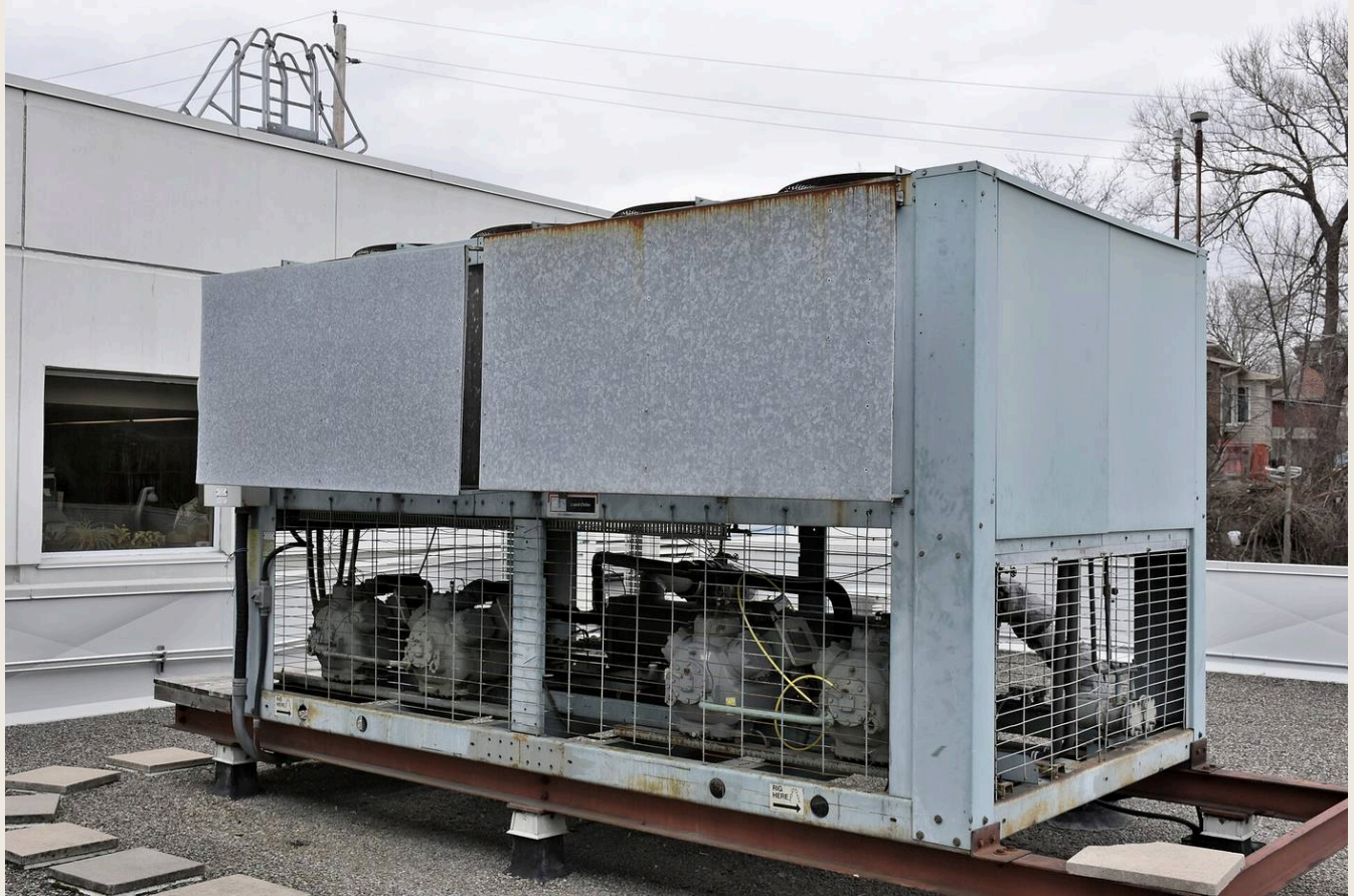
FIG. 04 · AIR-COOLED CHILLER ON INDUSTRIAL ROOF · PHOTO: SAUD / WIKIMEDIA COMMONS · CC BY-SA 4.0. Source and licence
