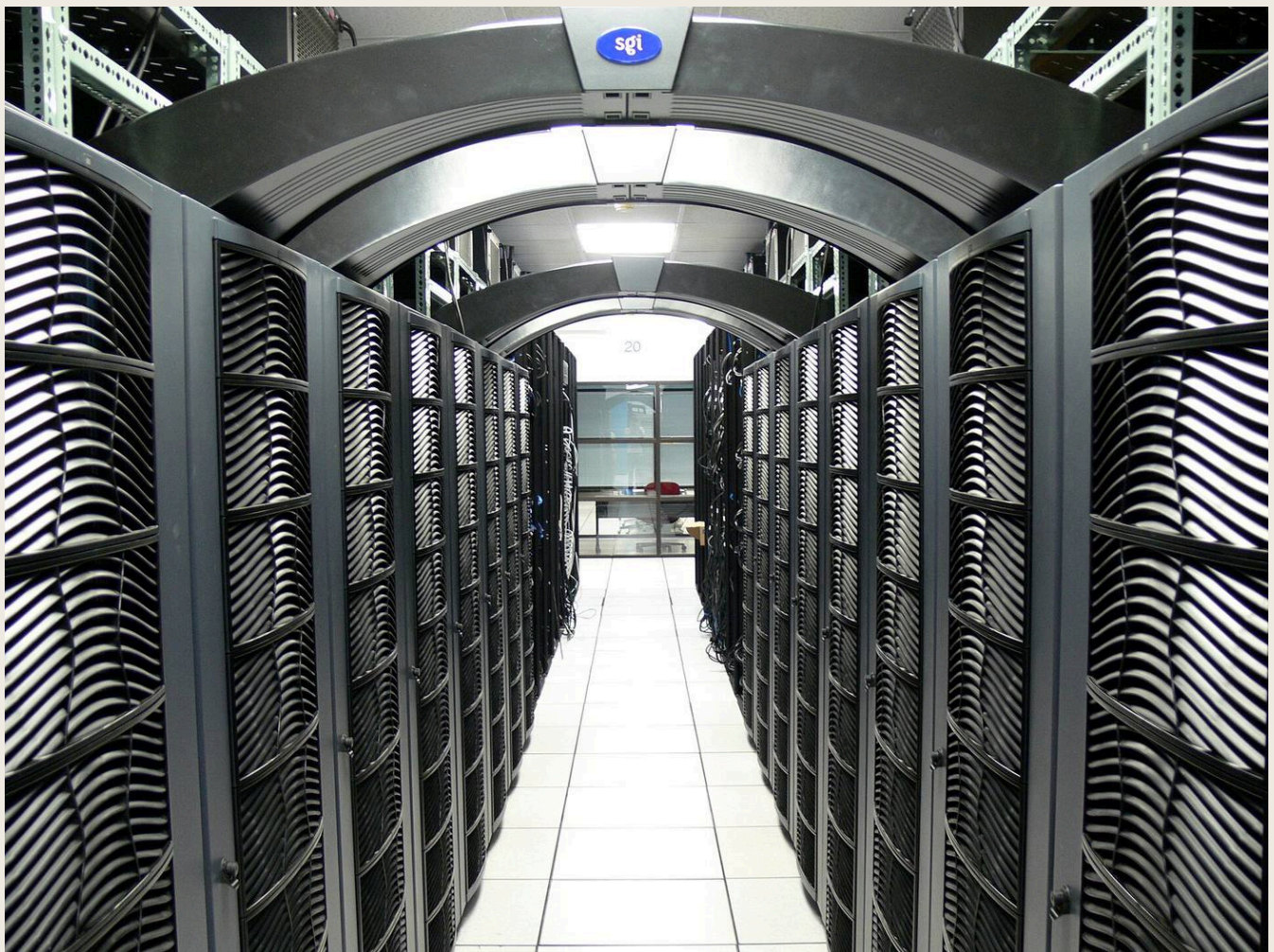
FIG. 09 · SERVER-HALL CORRIDOR, VIRGINIA TECH · PHOTO: CHRISTOPHER BOWNS / WIKIMEDIA COMMONS · CC BY-SA 2.0. Source and licence
