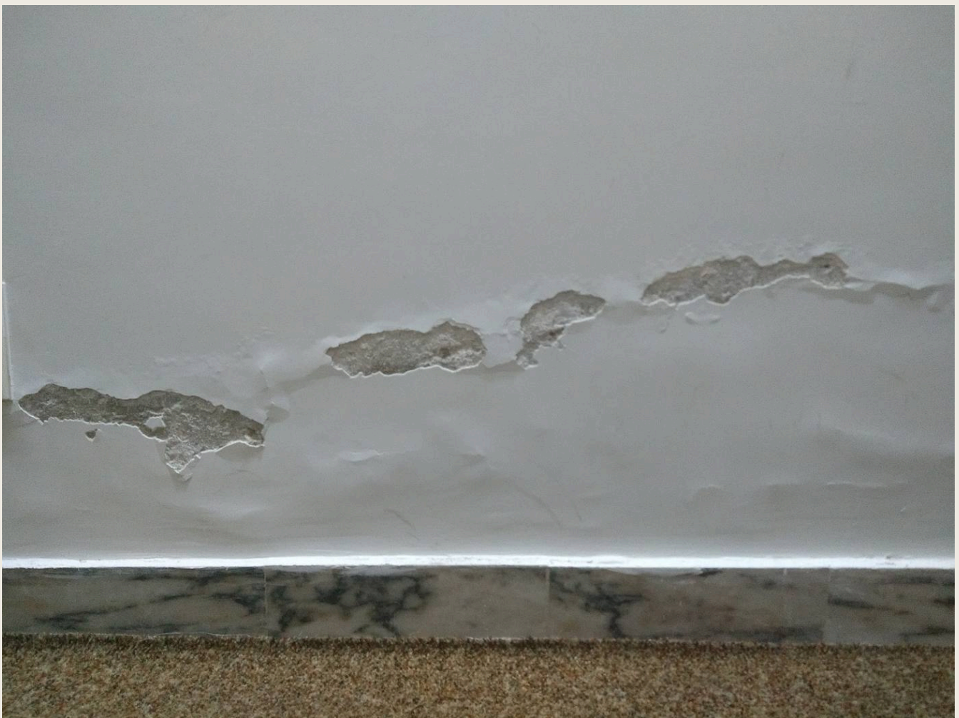
FIG. 08 · RISING DAMP ON AN INTERNAL WALL · PHOTO: Kebabknight / WIKIMEDIA COMMONS · CC BY-SA 4.0. Source and licence
