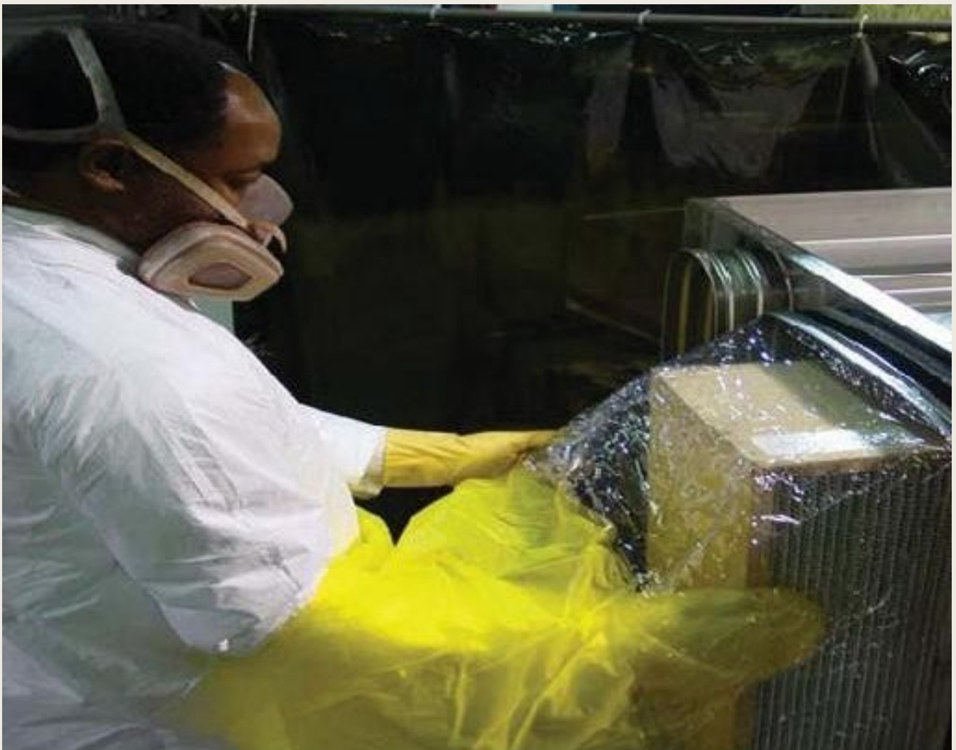
FIG. 22 REMOVING A DIRTY FILTER FROM A VENTILATION UNIT · PHOTO: NATIONAL
