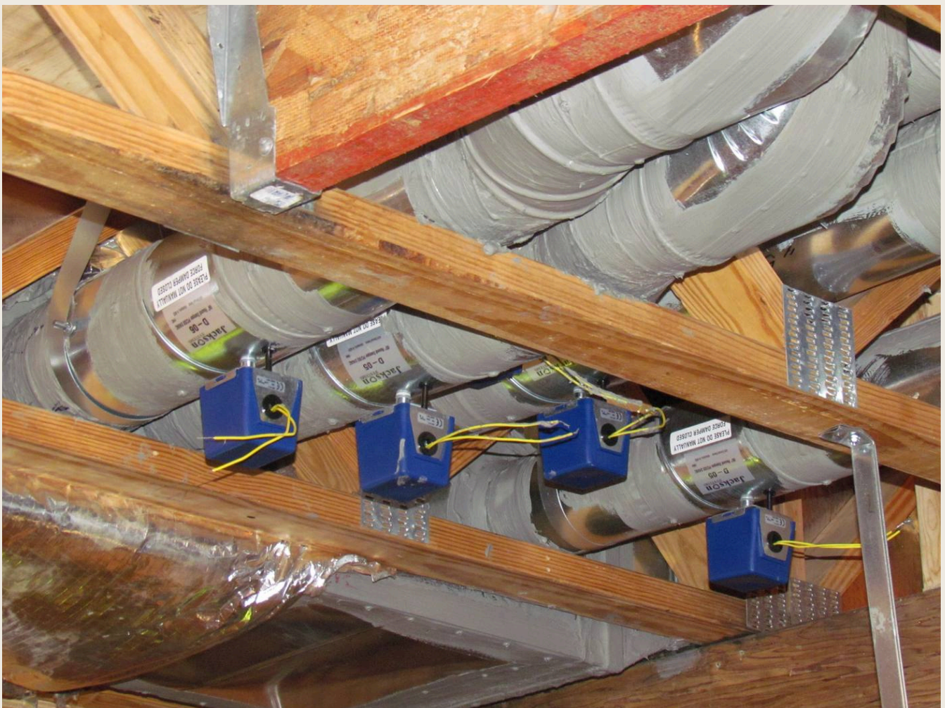
FIG. 08 · DUCTWORK IN A BASEMENT CEILING · PHOTO: NATIONAL INSTITUTE OF STANDARDS AND TECHNOLOGY / WIKIMEDIA COMMONS · PUBLIC DOMAIN (US FEDERAL). INSTALLED DUCTWORK, NOT THE ACT OF INSTALLATION. Source and licence
