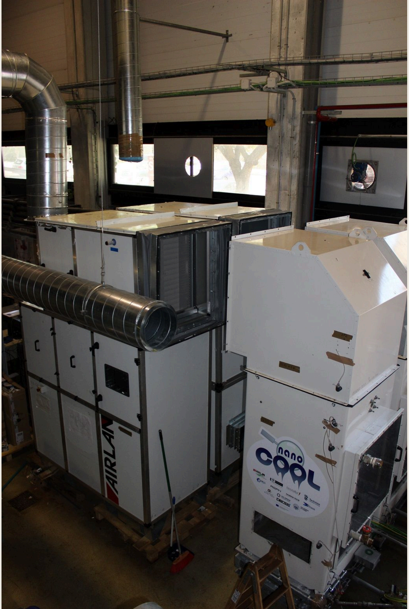
FIG. 01 · AIR HANDLING UNITS · PHOTO: NANOCOOL PROJECT / WIKIMEDIA COMMONS · CC BY 3.0. Source and licence
